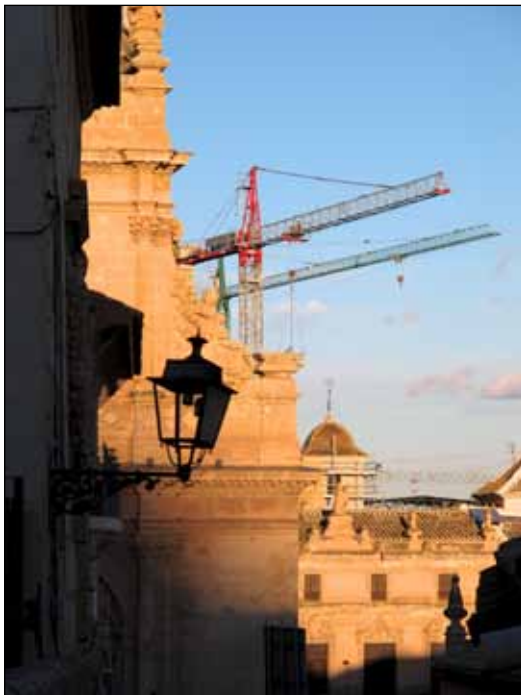
Repairs underway after the 2011 earthquake, to Lorca's historic buildings in the town below the castle.
