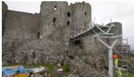
Harlech Castle. New footbridge being installed during redevelopment works at the site.
