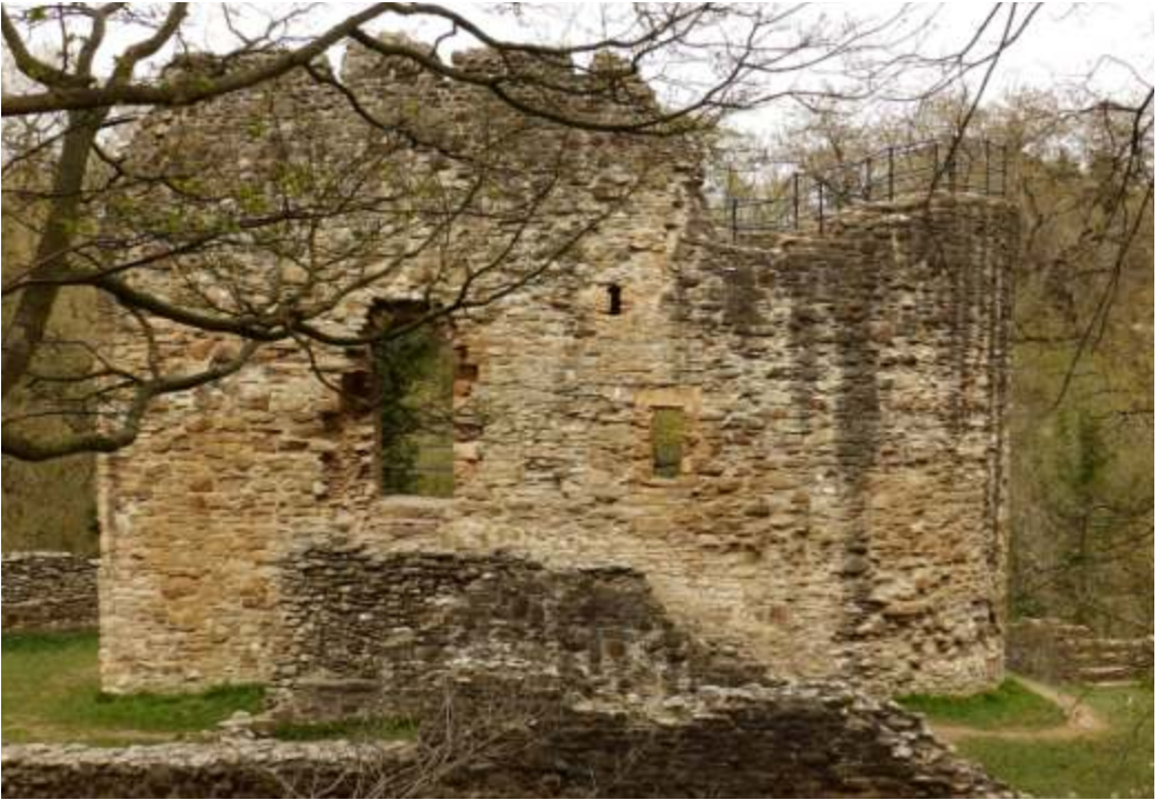
ABOVE: Entrance forebuilding/staircase leading to the first floor entrance and a further set of straight stairs within the thickness of the wall up to the battlements.
