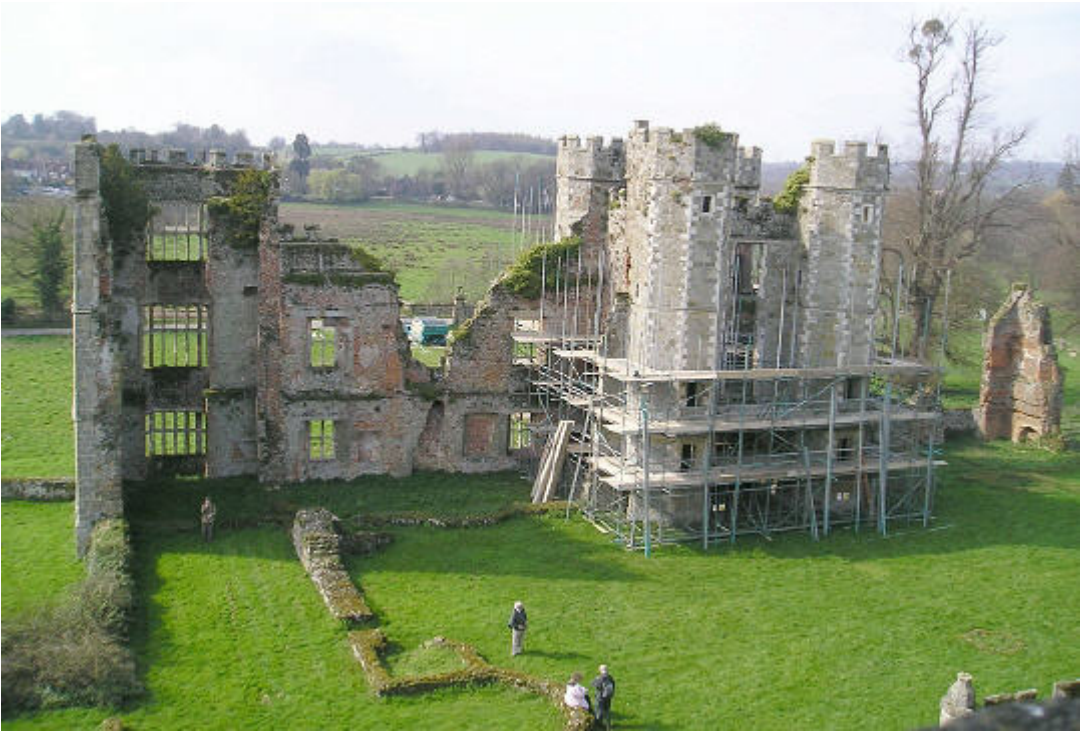
Fig 22 Cowdray House. To the left is the demolished south range . Centre right the west range gatehouse. The south range originally contained a long gallery at first floor level, to mirror that on the north range. It was later altered into accommodation units.
