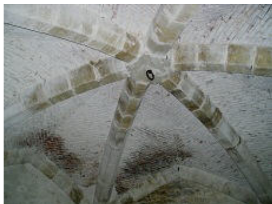
Fig 20 Cowdray House. The rib vaulted chamber or cellar of the hexagonal strong tower, built circa 1520-30's which housed the bedchamber of the Earl.
